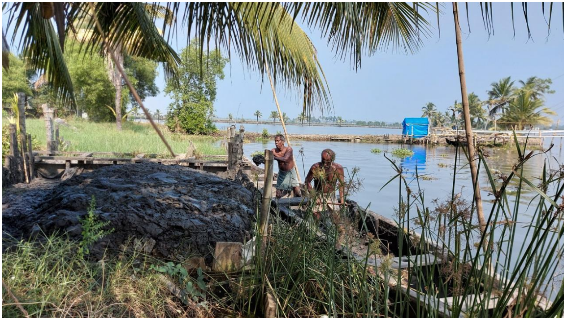
Figure 9. Dredging Mud from the Backwaters, to Elevate Field Bunds at Ezhikkara, Ernakulam
