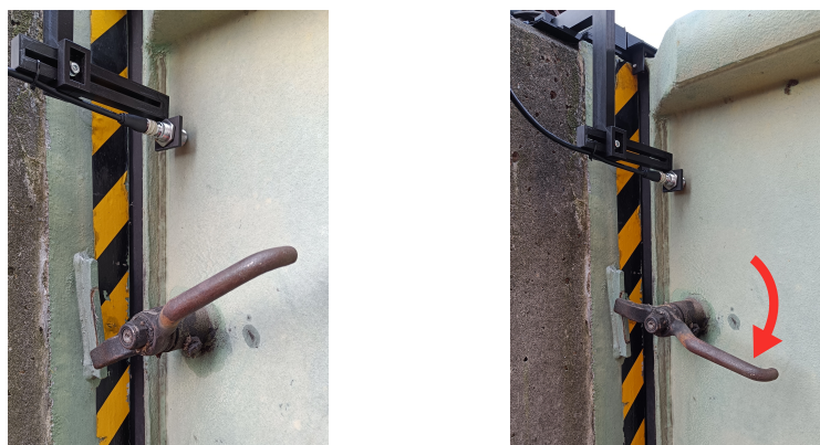
Figure 18. Deployment test of the inductive sensor to correctly detect the final closing positions of the gate.
