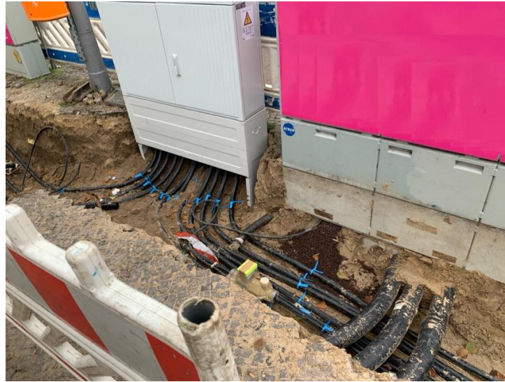
Figure 6. Distribution Cabinets connecting electricity network and data networks
